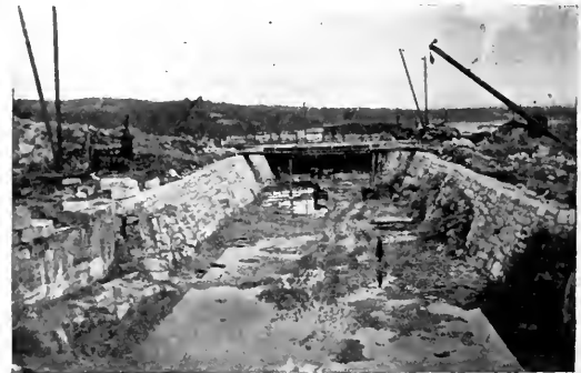
FIG. 5.—CANAL FROM HEAD GATES, GARVIN'S FALLS.
